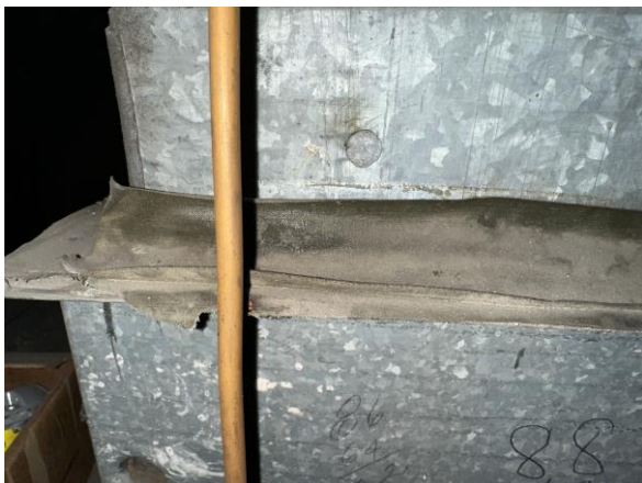
Photo 11 HA-12: Black HVAC seal
