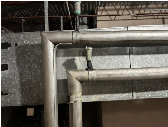
Photo 9 HA-10: Black asphalt patching at pipe connection joints
