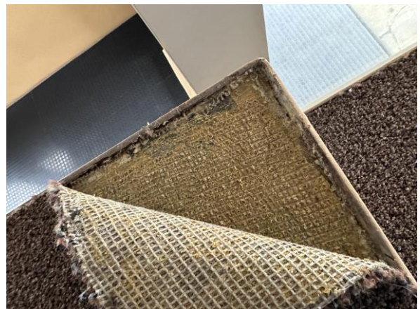
Photo 12 HA-13: Yellow carpet mastic (stairwells)
